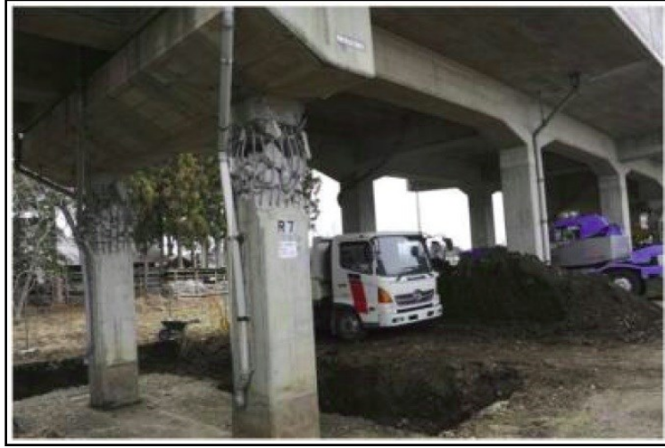
Figure 6-1: Nakasone Viaduct after the 2011 Great East Japan Earthquake (Kawashima et al. 2011)
